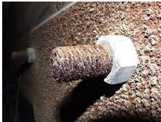
Figure 1.5 : Corrosion frottement (tribocorrosion).
